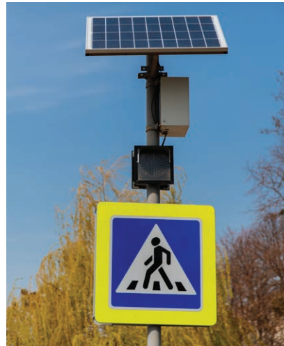
Small scale solar application
