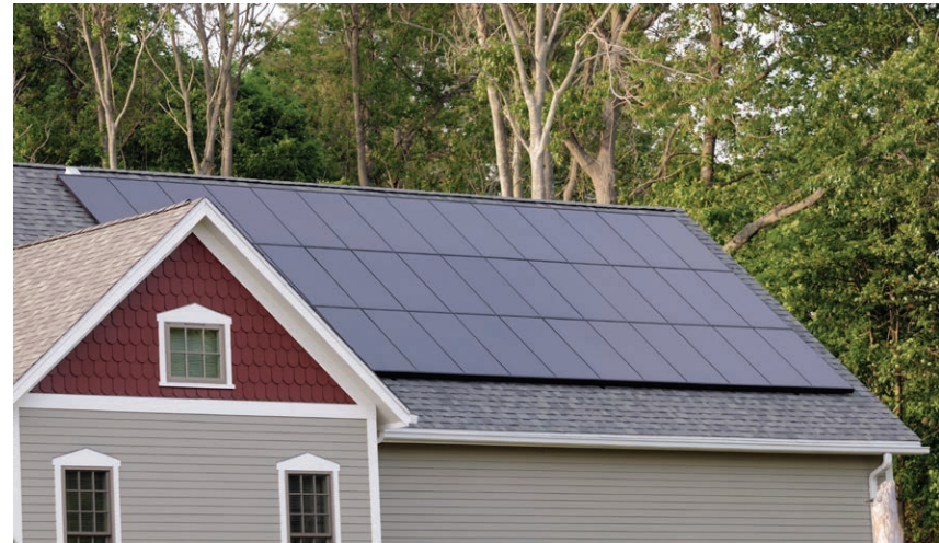
Residential scale solar application
