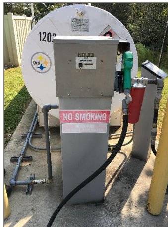
Fuel Station and Pump
