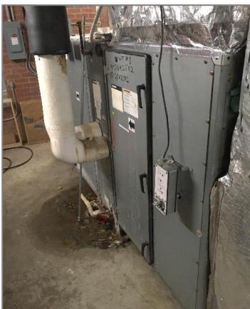
1 st Floor Air Handler
