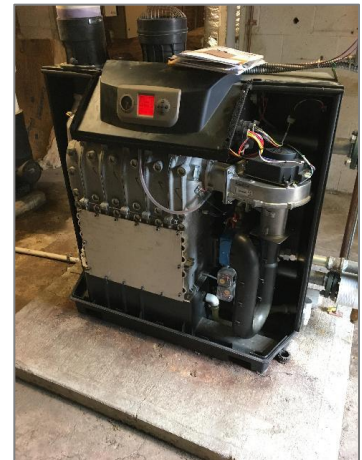
1 st Floor Boiler for HVAC
