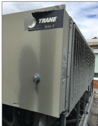
Chiller for HVAC
