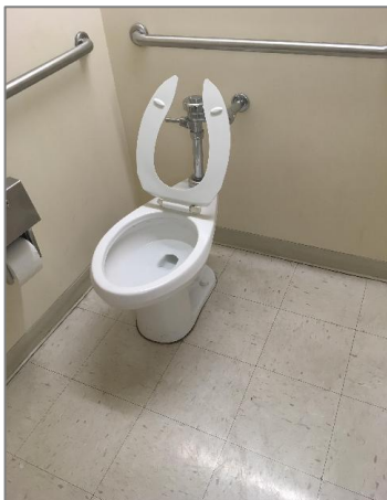
Water Closet (fixtures)
