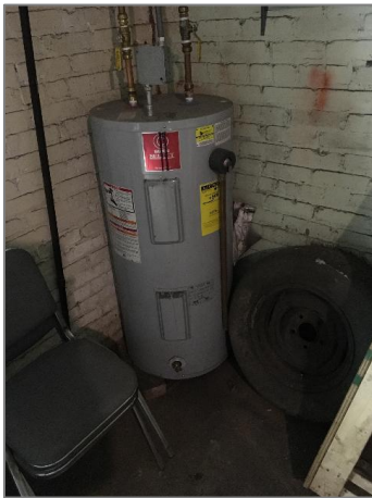
Hot Water Heater
