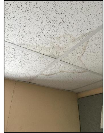
Damaged Ceiling Tiles
