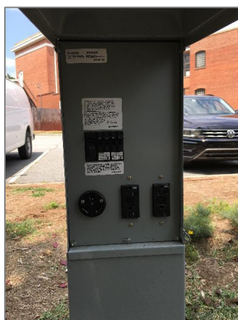
Power Pole Box
