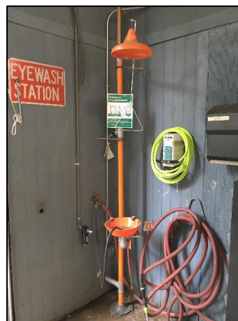
Eye wash Station
