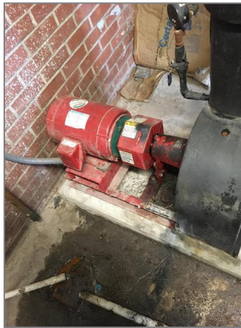
Hot Water Pump for HVAC
