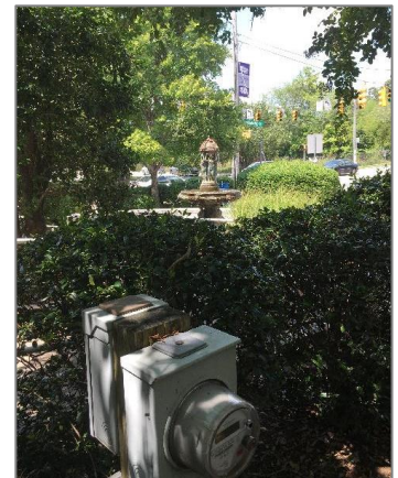
Statue, Fountain, and Electrical Panel
