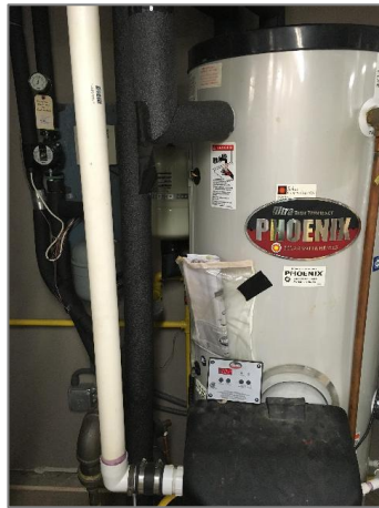
Solar Hot Water Heater
