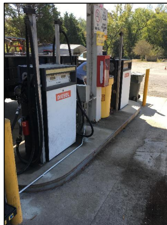
Fuel Pump Station
