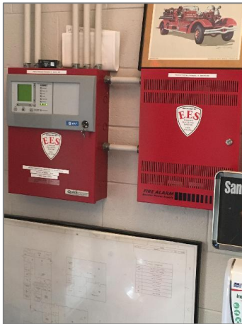
Fire Alarm System
