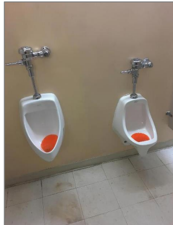
Water Closet (fixtures)
