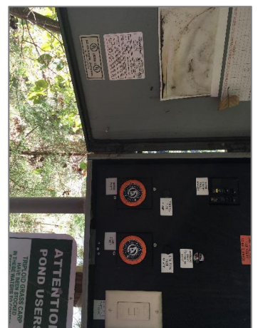
Electrical Panel (Near Pond)
